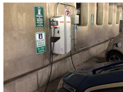
Two of Eastern's electric charging stations in Shakespeare Garage
