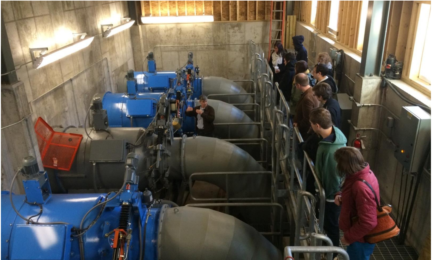
The mid 1800's dam has been converted to hydroelectric providing up to 500 kW of clean renewable energy through four turbines.
