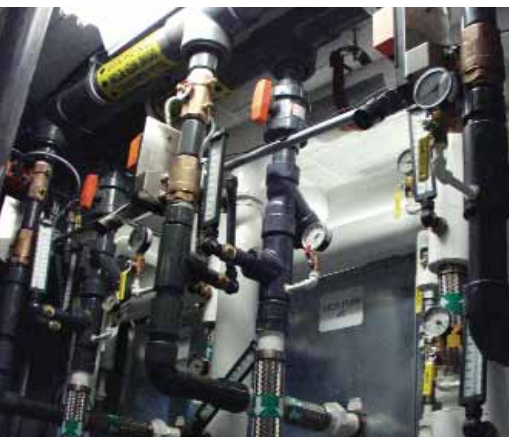
[below] geothermal energy pipes.
