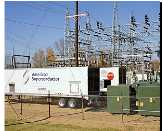
Power Electronic Systems
