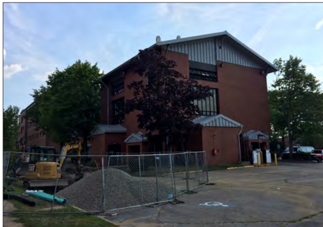
Existing Central Plant
