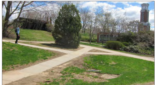
Opportunistic desire line diagonals have resulted in incremental expansion of pavements, and attendant compaction and snow management damage.
